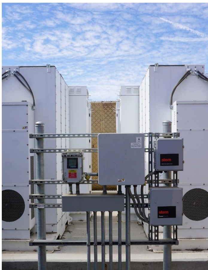
An example of a Stem battery storage system installed at a commercial building Permission granted by Stem
